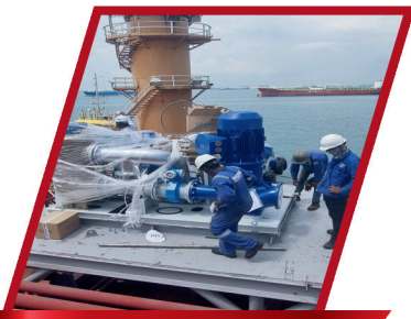
BWTS & Electrical Installation
