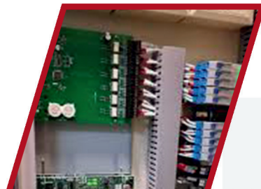
Fire & Gas Detections
