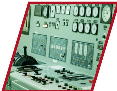
Switchboard & Control Panel
